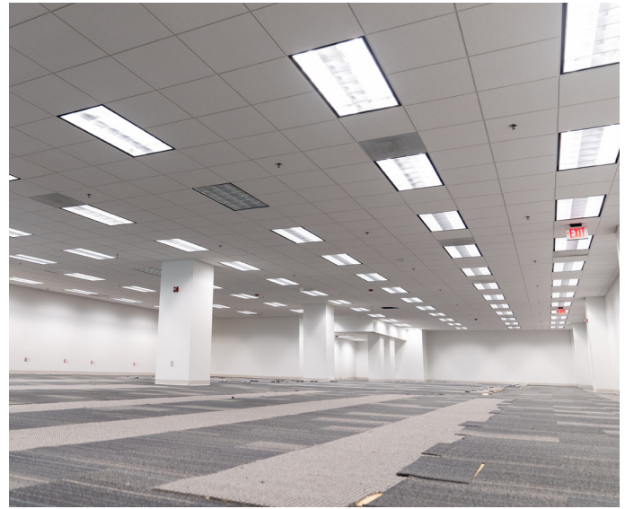
Since FY 2021, the USPTO has reduced the physical footprint of its Alexandria headquarters and adjacent facilities by approximately 1 million square feet. (Photo by Michael Connor/USPTO)
